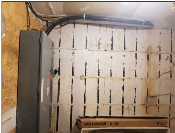
Photo 4.1.1.1-1 Water penetration at electrical conduit
