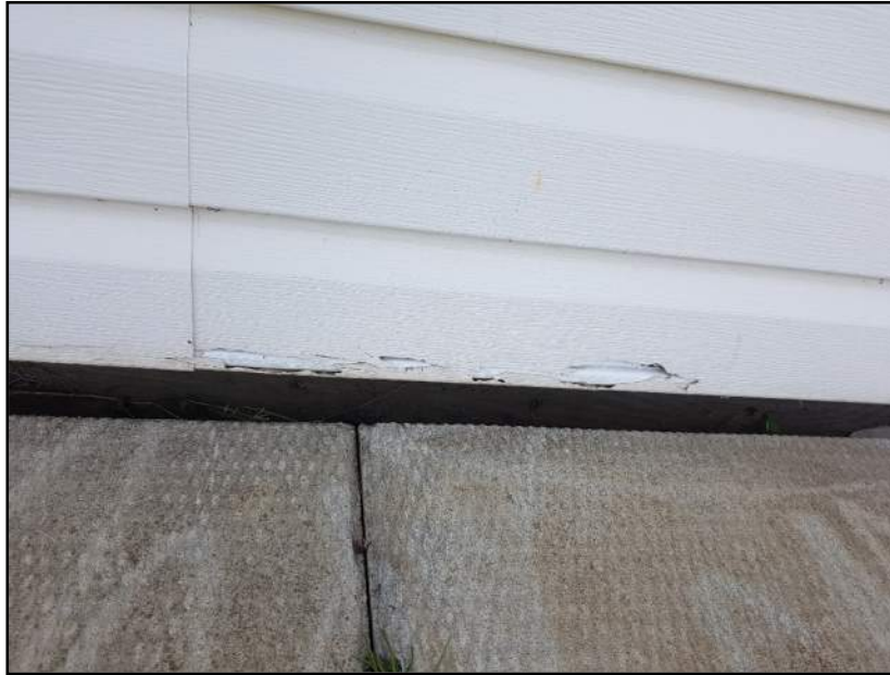
Photo 4.2.1.1-2 Typical damaged vinyl siding
