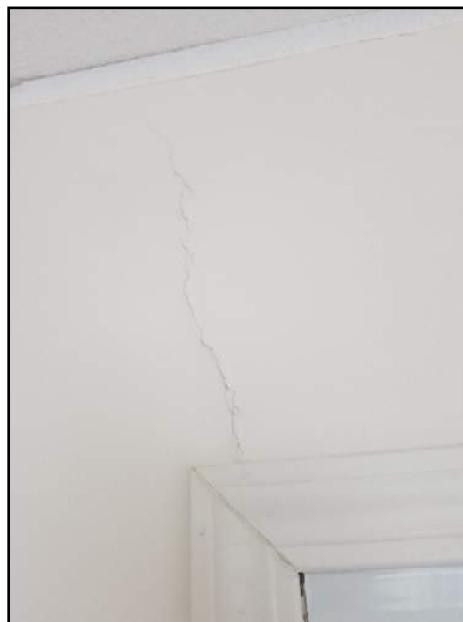
Photo 4.1.2.1-3 Crack in gypsum at door head
