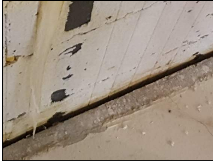
Photo 4.1.1.2-2 Gap between foundation wall and slab-on-grade
