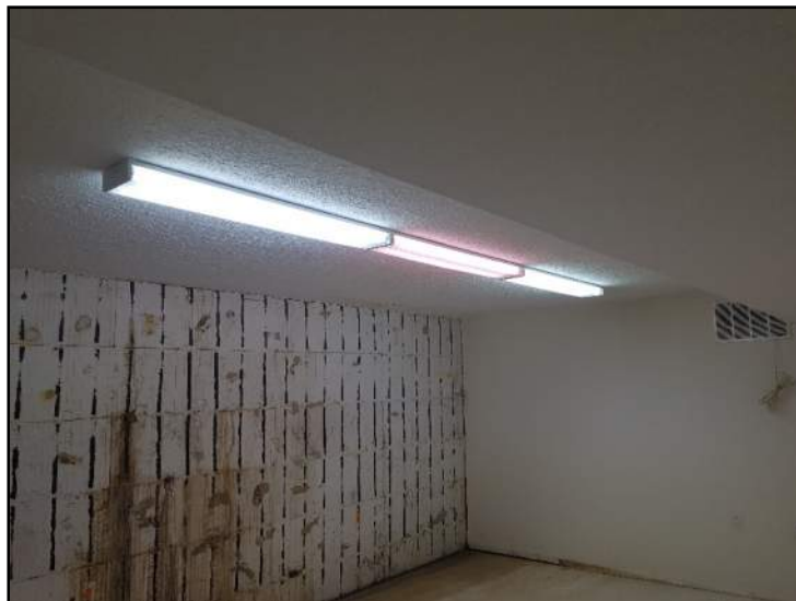
Photo 4.5.5.1-1 Typical strip fluorescent fixtures
