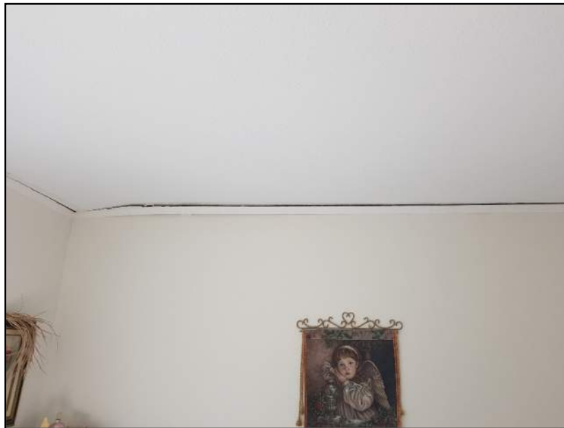
Photo 4.1.2.1-1 Ceiling gap between unit 3 and 5
