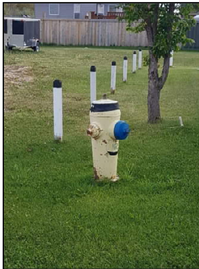
Photo 4.6.1.1-1 Typical fire hydrant
