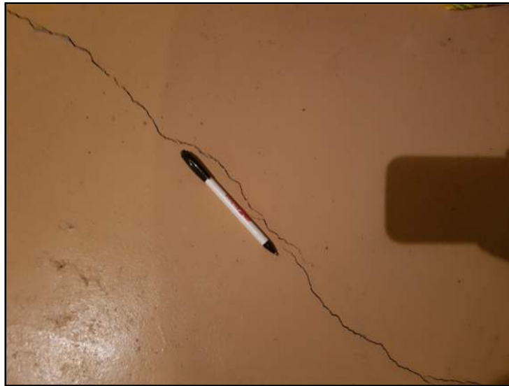
Photo 4.1.1.2-1 Typical crack on slab-on-grade
