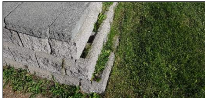
Photo 4.7.4.1-2 Shifted stacked stone retaining wall
